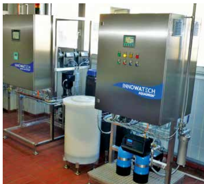
INNOWATECH HyClean plus Concept® spray system and Aquadron® SGX serve well and reliably at a renowned Bavarian brewery.
