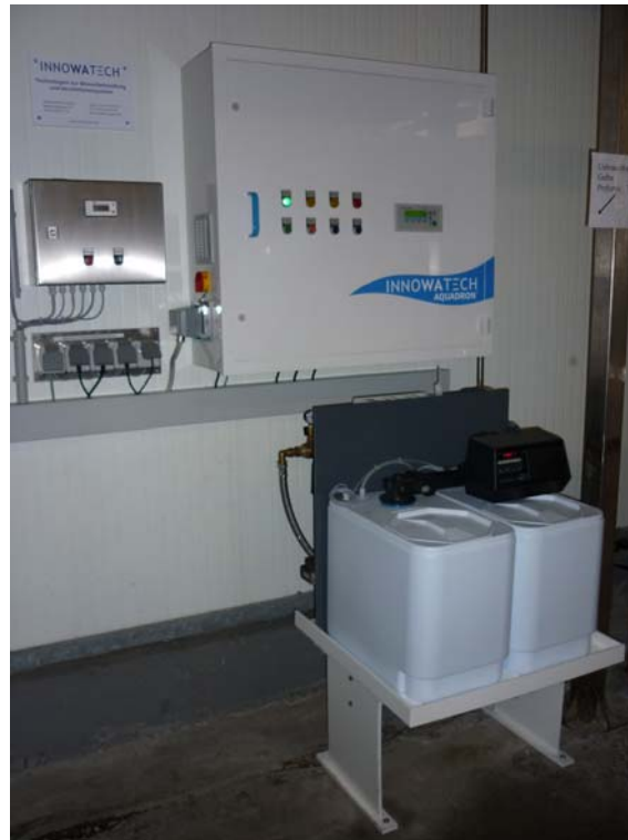
Abb. 2: INNOWATECH Aquadron® Anlage
